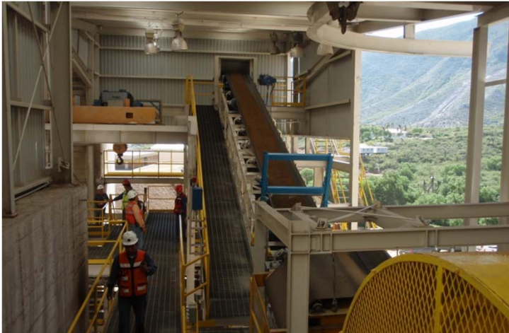
Secondary/Tertiary Crusher Plant
