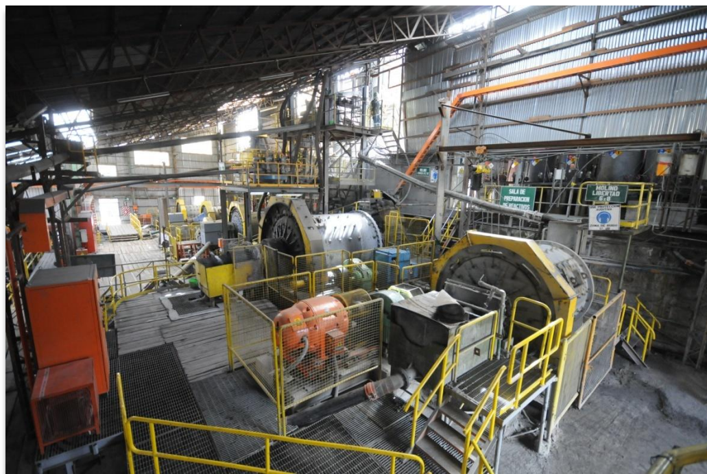
CAYLLOMA MINE: 1,250 tpd processing plant
