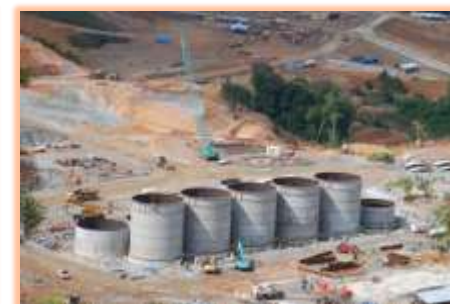
*CIL Tank Area at Plant Site
