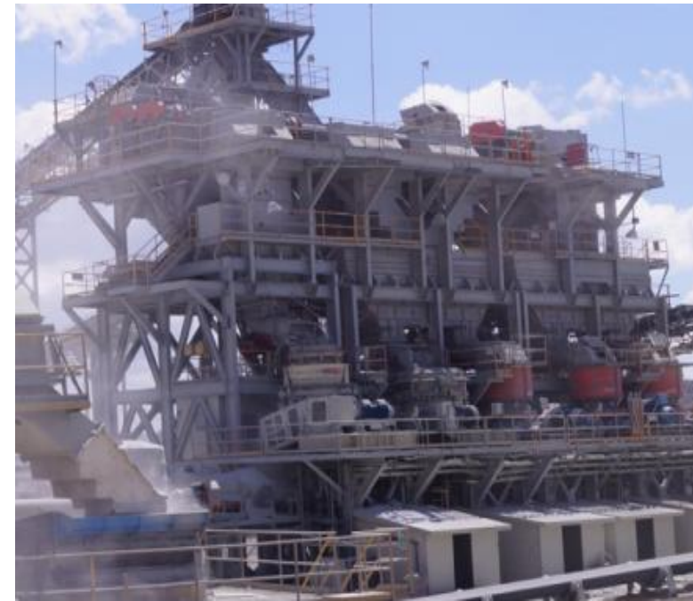
New crushers installed for throughput of 24,000 tpd
